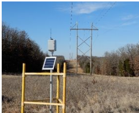
Figure 4: LineVision PACT monitor installed in the field.
